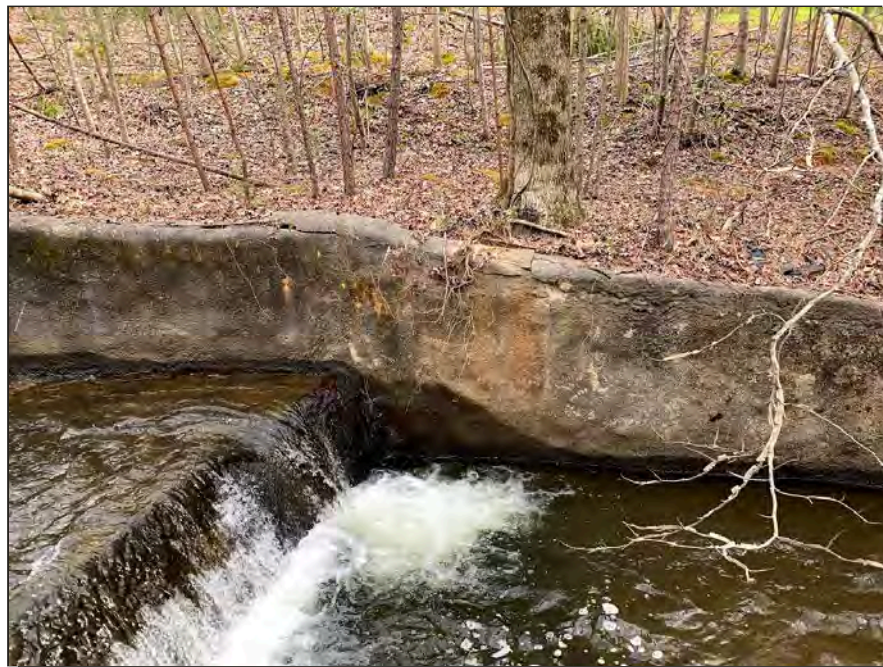
Photograph 26: Spillway, 2020 – general view of cracking on the sides of the spillway near tree roots.
