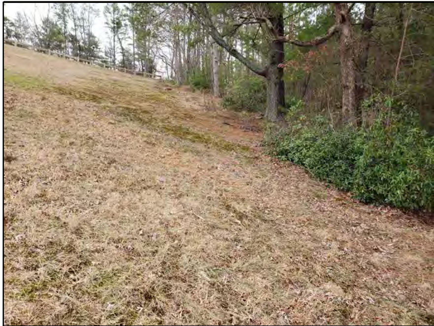
Photograph 11: Downstream Face, 2020 – typical surface erosion observed along the left abutment.
