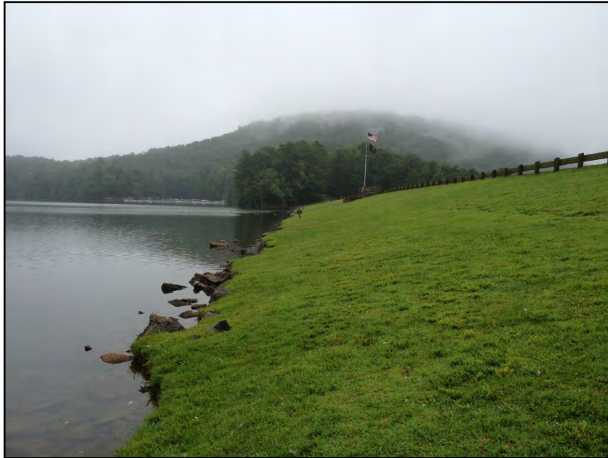
Photograph 1: Upstream Face, 2013 – localized areas of erosion and beaching along shoreline.
