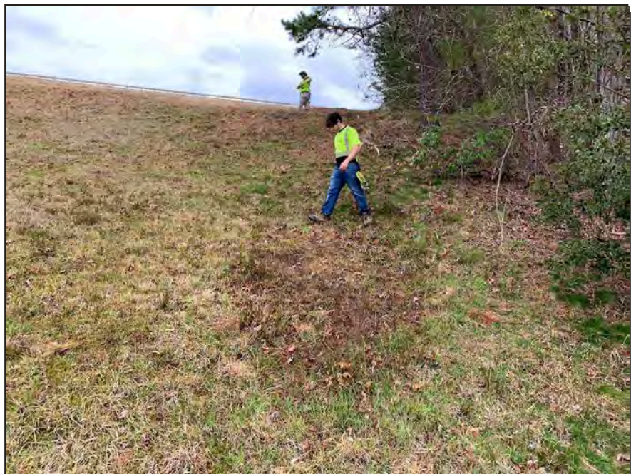
Photograph 18: Downstream Face, 2020 – wet surface area found between downstream benches.
