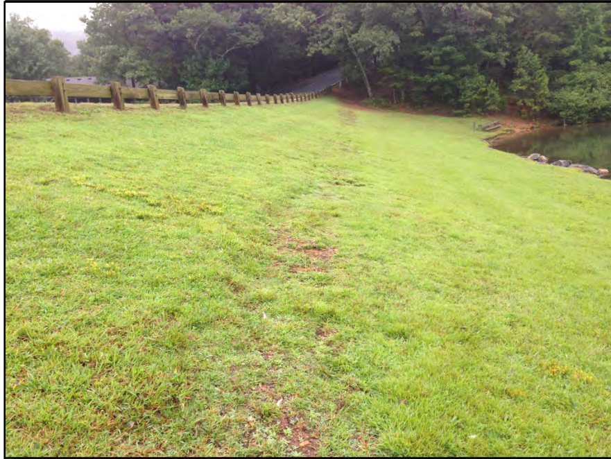
Photograph 3: Upstream Face, 2013 – slope surface erosion midway up the western half of upstream face.
