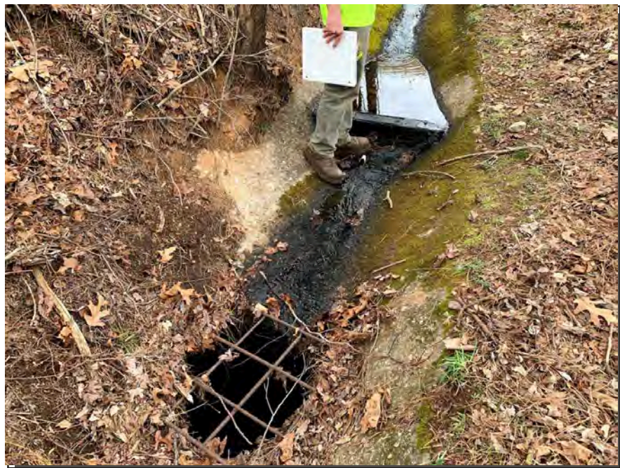
Photograph 16: Downstream Face, 2020 – the drop inlet on the right abutment was generally clear of sediment and debris.
