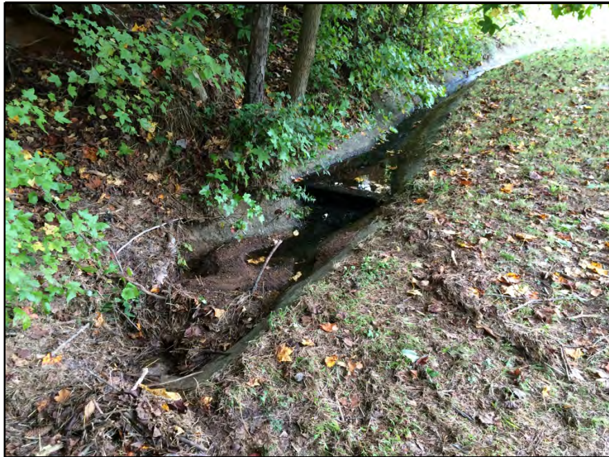
Photograph 15: Downstream Face, 2014 – sediment and debris accumulated at the end of the concrete channel, partially obstructing the drop inlet at this location on the right abutment.
