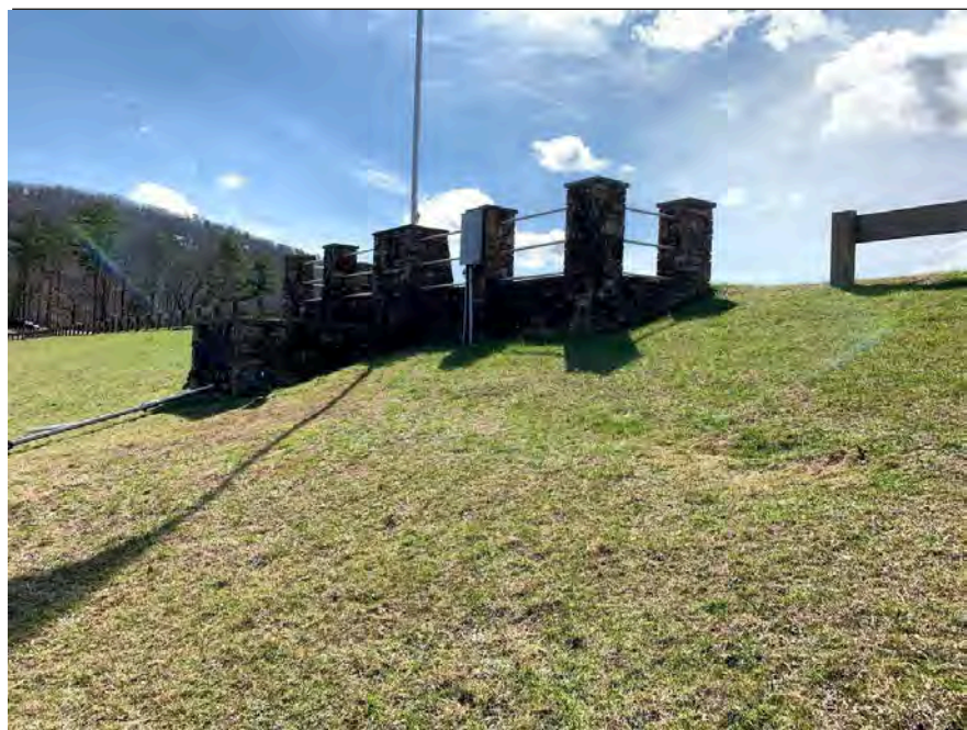
Photograph 8: Upstream Face, 2020 – surface erosion decreased around valve box.
