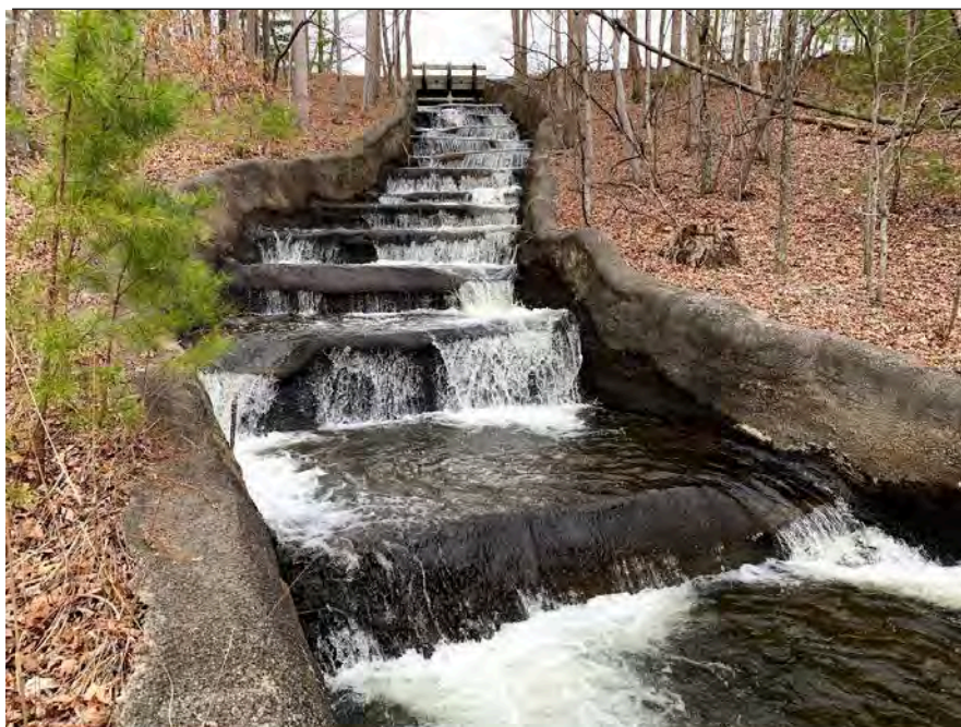
Photograph 24: Spillway, 2020 – general view of stepped spillway with moderate flow, and tree limbs and debris noted during inspection.
