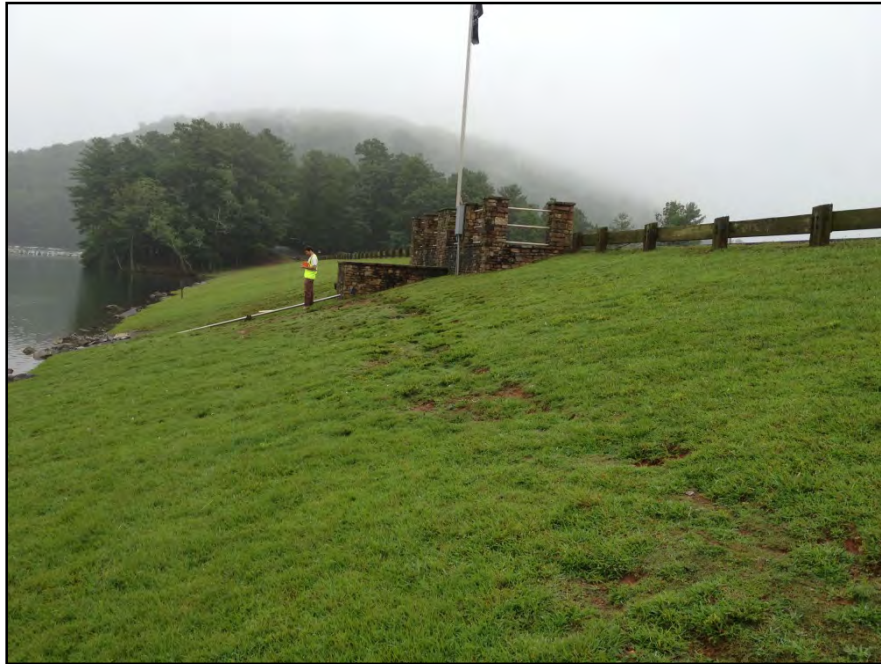
Photograph 5: Upstream Face, 2013 – slope surface erosion midway up the western half of upstream face.
