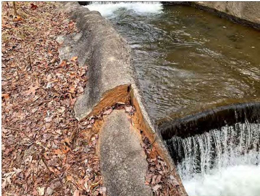
Photograph 25: Spillway, 2020 – general view of broken area on the side of the spillway with moderate flow during observation.
