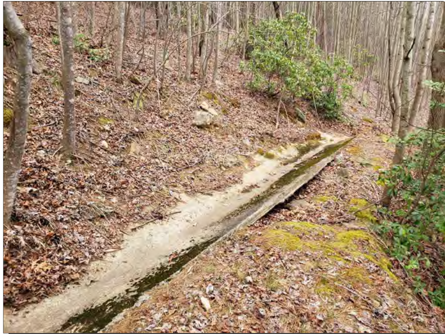
Photograph 17: Downstream Face, 2020 – concrete channel eroding underneath on left abutment.
