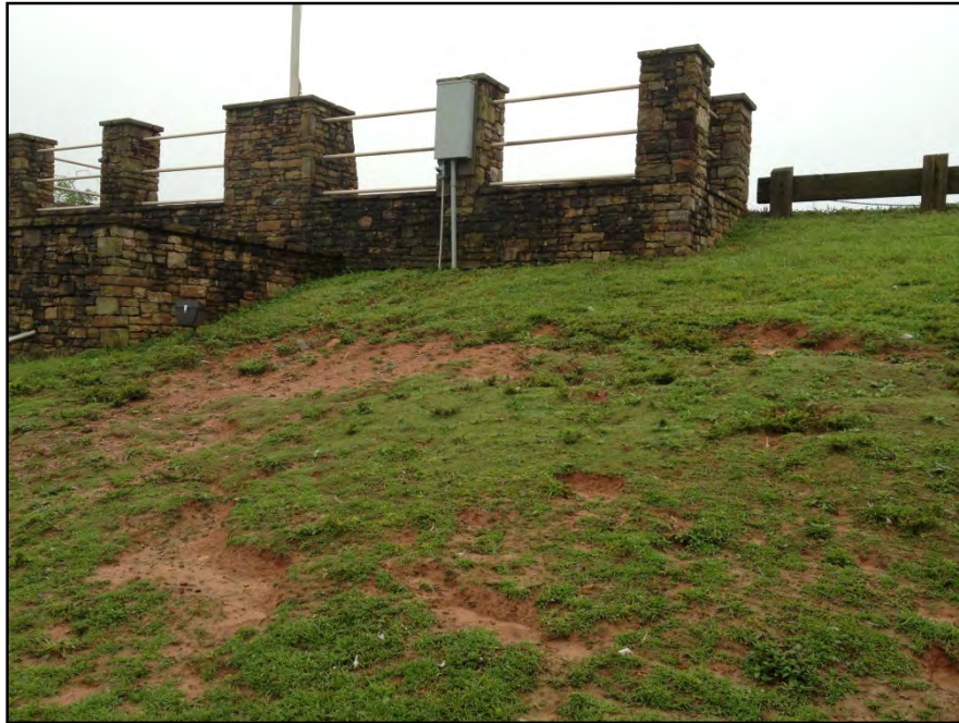
Photograph 7: Upstream Face, 2013 – surface erosion around valve box.
