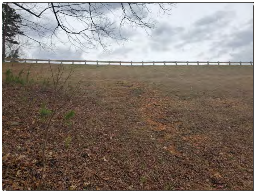
Photograph 12: Downstream Face, 2020 – surface erosion observed on the right abutment between benches.
