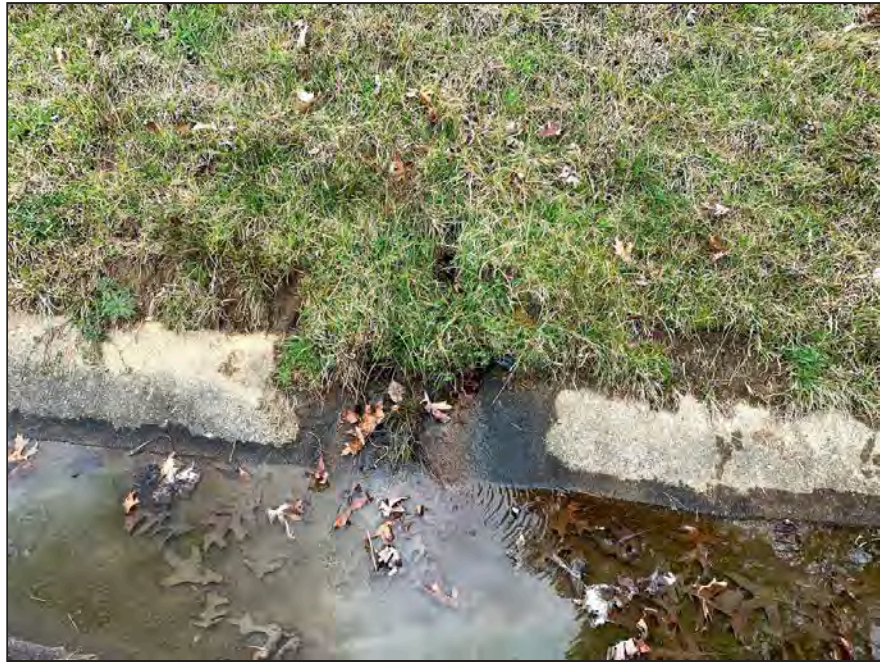
Photograph 19: Downstream Face, 2020 – clogged interceptor drain with low flow.
